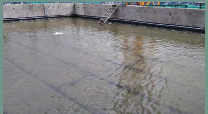
Pictured Above: Example of roof flood
